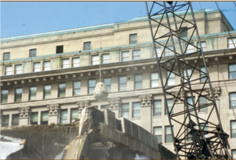
A close-up view of the wrecking ball just before it makes impact with the reinforced concrete garage.
