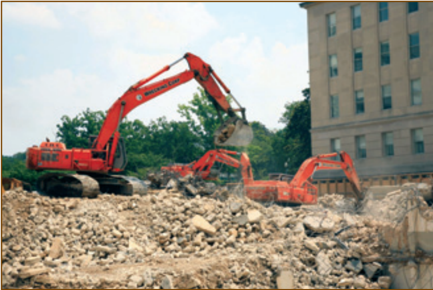
Two of the excavators are equipped with pulverizers and one with a bucket and thumb in order to break up the concrete. Photo by James Tetro.
