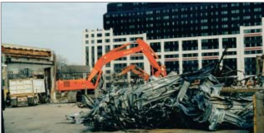
Demolition of the former Washington Convention Center is just the latest high-profile job for Wrecking Corporation of America. Here, a Wrecking Corp. operator uses a Hitachi Zaxis 450 to sort and separate material.
