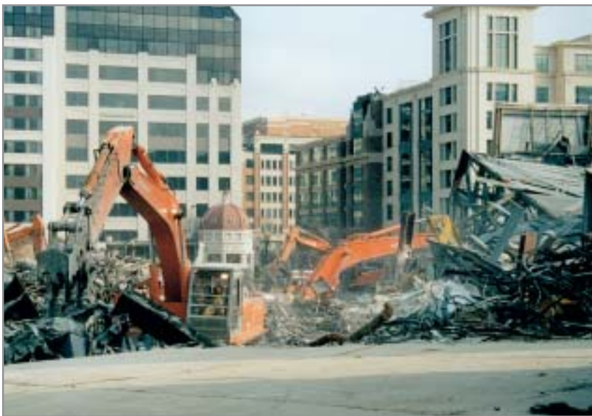
Wrecking Corporation of America imploded the Washington Convention Center on Dec. 18, 2004. Cleanup is expected to be complete by the end of June 2005.
